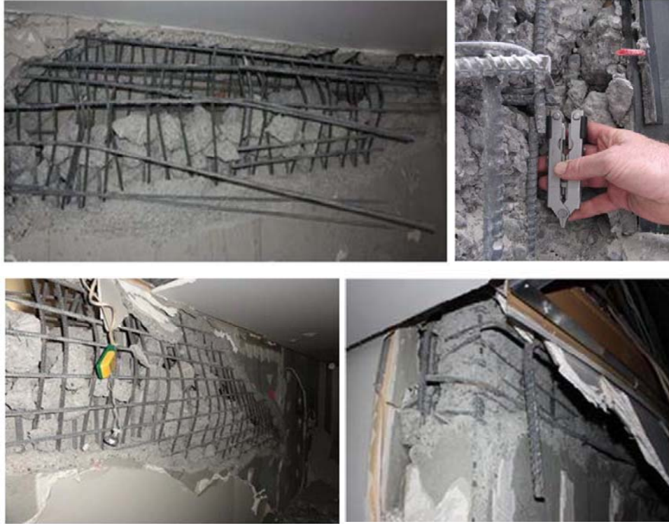
Figure 1-1. Typical brittle wall failures in 2011 Christchurch earthquake (Sritharan et al. 2014)
