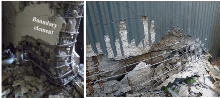
Figure 1-2. Damage in plastic hinge region, 2011 Christchurch earthquake (Sritharan et al. 2014)
